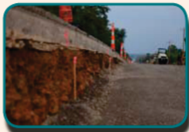
Construction progress continues on 141st St. S. This widening project will address the growing traffic needs in the Jenks/Glenpool area.
